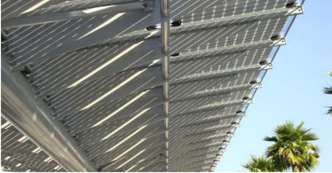
Fig. Onyx Solar Photovoltaic Canopy System installed at Bart Station, San Francisco, CA . Peak Power: 164 kWp stc ~ 149 kWh ptc.
